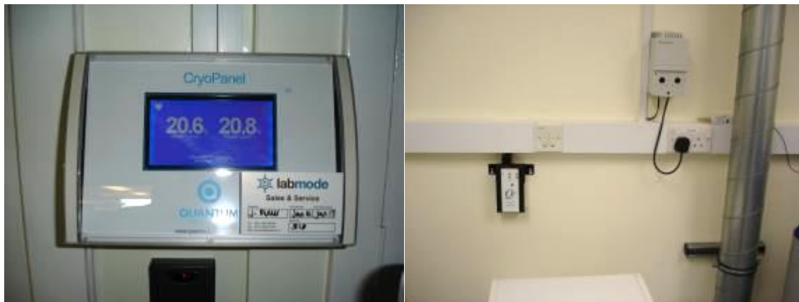
Figure 2: Control panel for O2 levels & Example of O2 sensor in repository
