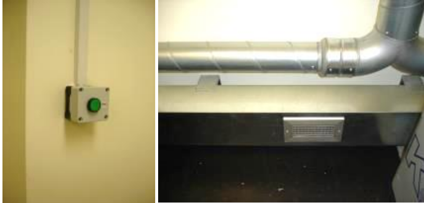
Figure 4: Fan override button and fan air entry vent
